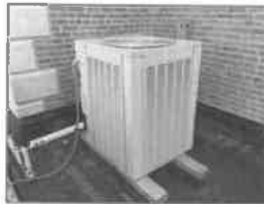
AC Condensing Unit
