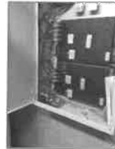
Building Automation Control Panel
