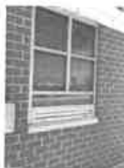
Window With Louver
