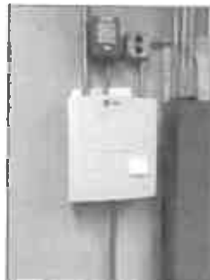
Trans Control Panel
