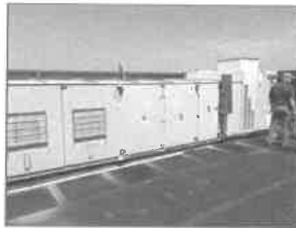
Trane Rooftop Unit
