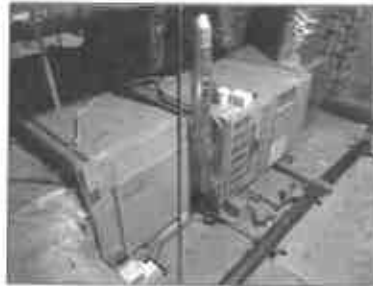
Furnace in Attic
