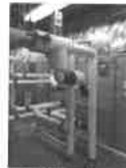
1994 Air Handling Unit
