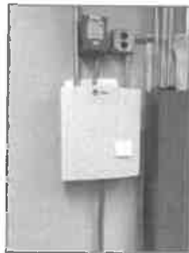
Trans Control Panel
