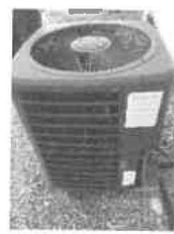
Condensing Unit Serving Office
