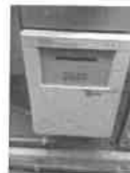
Term Control Panel
