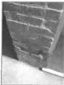
Exterior Brick Deterioration
