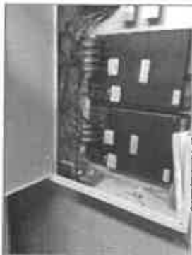
Pneumatic Control Panel
