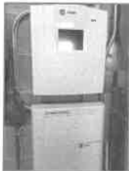
Trane Control Panel
