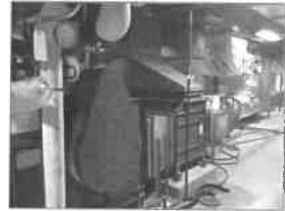
VAV Air Handling Unit
