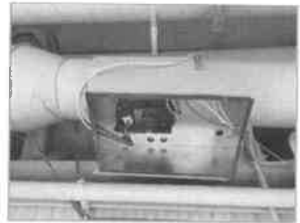
VAV Box Controller
