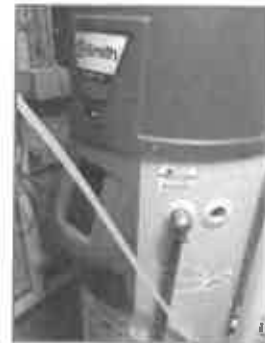
High Efficiency Water Heater
