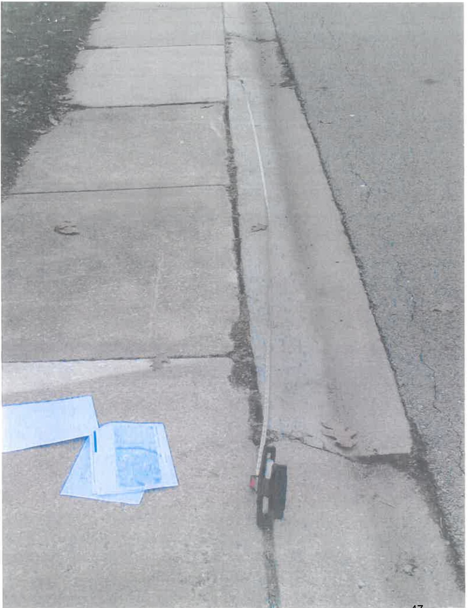
Pavement and Sidewalk Separated by Black MAT Expansion JOINT 47 NOT ONE
