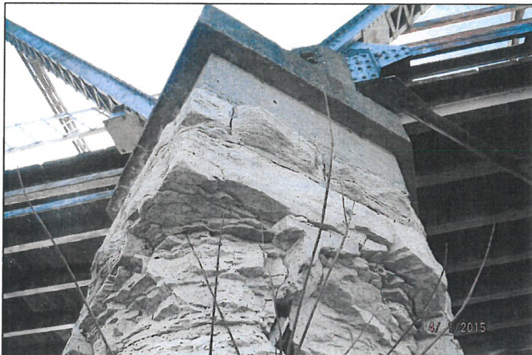
Photograph 20: View of Section Loss at the Upstream Nose of Pier 1, Looking Upward.
