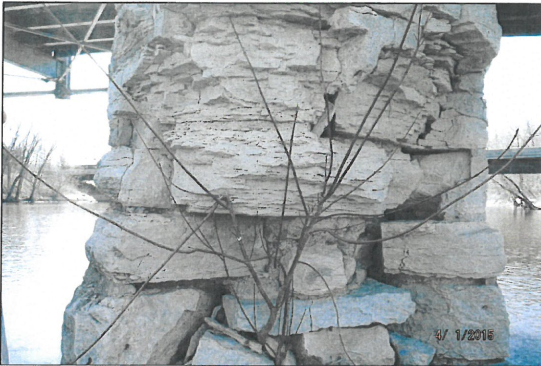
Photograph 19: View of Section Loss at the Upstream Nose of Pier 1, Looking South.
