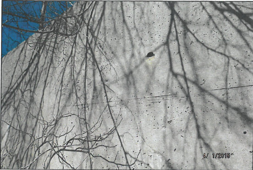
Photograph 11: View of Crack at the Downstream Wingwall of the West Abutment, Looking Northwest.
