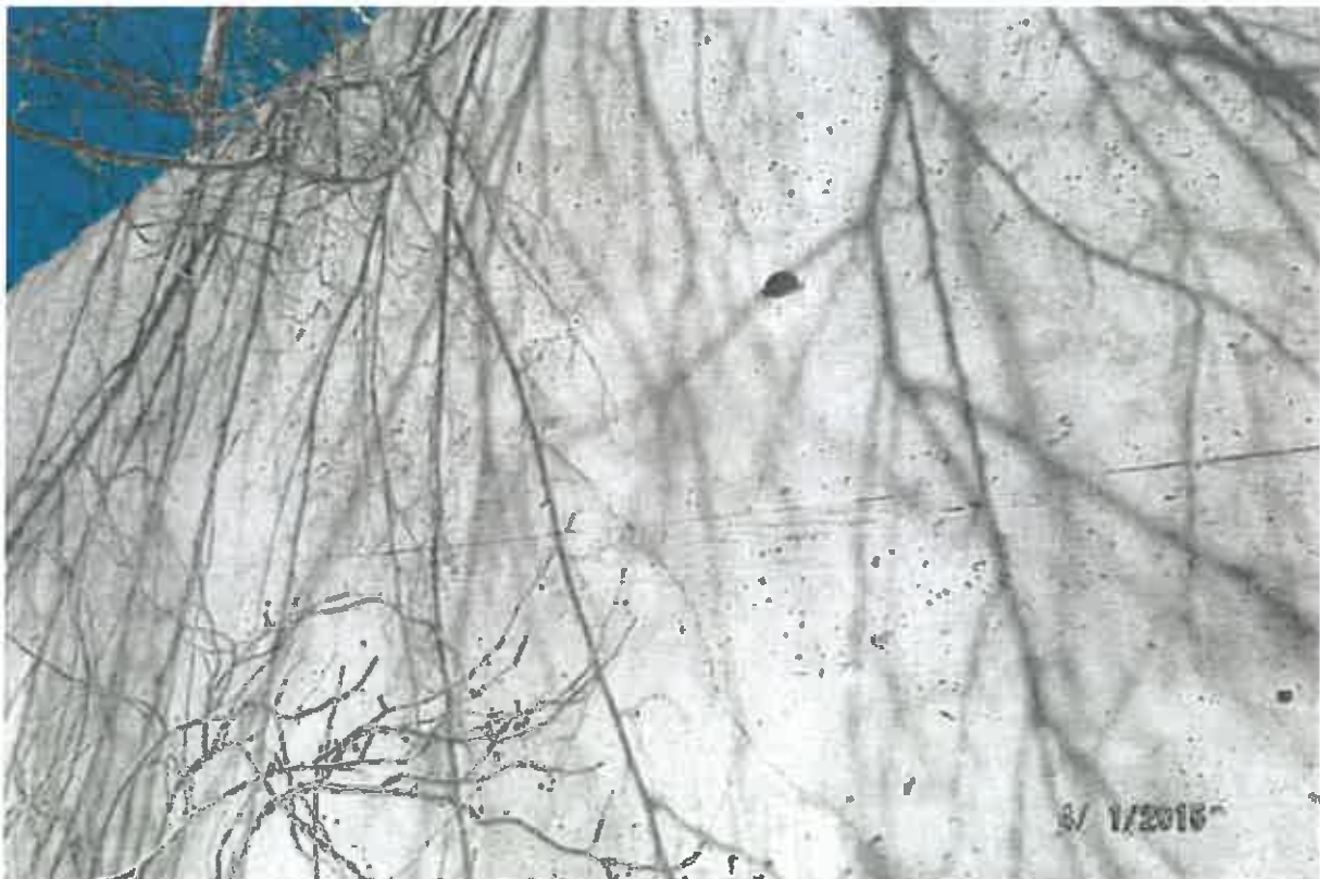
Photo 16_View of Crack at Downstream Wingwall of West Abutment, Looking Northwest-April 2015
