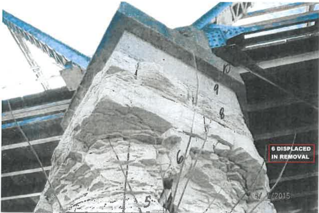
Photo 17_View of Section Loss at Upstream Nose of Pier 1, Looking Upward-April 2015
