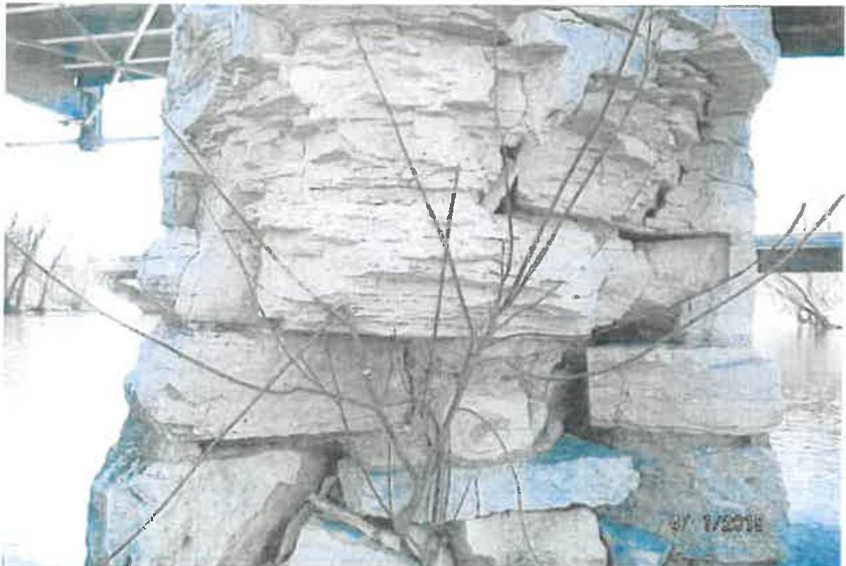
Photo 18_View of Section Loss at Upstream Nose of Pier 1, Looking South-April 2015
