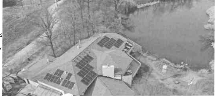
17.6kW Solar PV System on Emily Oaks Nature Center of Skokie Park District
