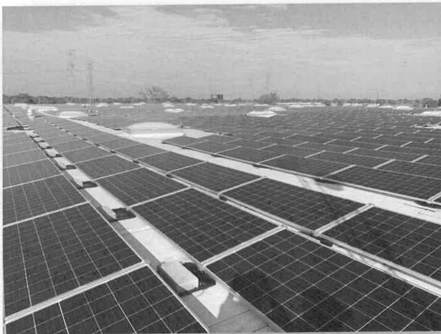
Roof Mounted in Illinois
