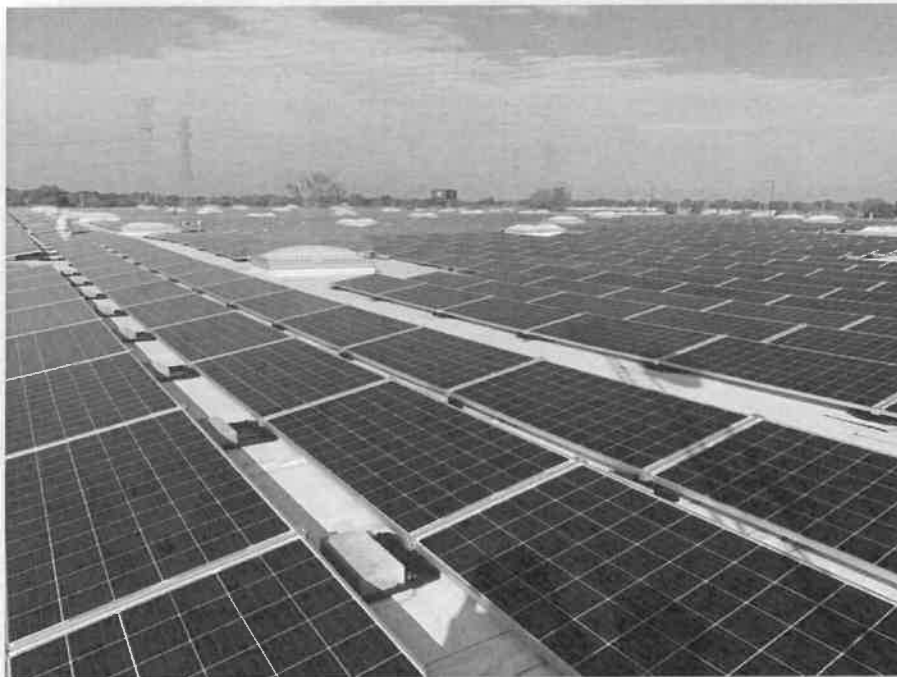
Roof Mounted in Illinois
