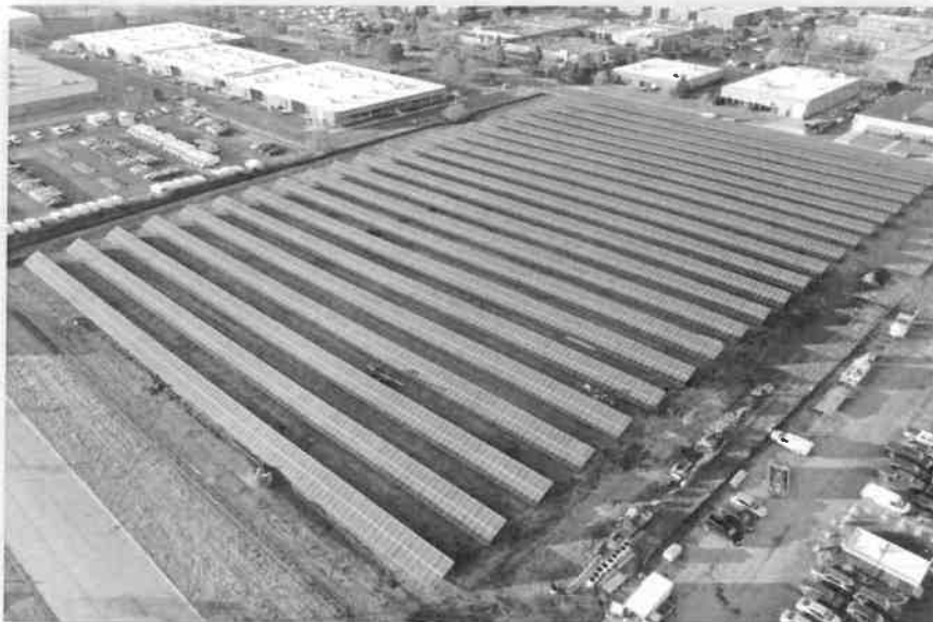
Ground Mounted in Illinois
