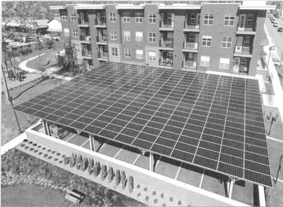
Canopy / Carport Mounted in Indiana
