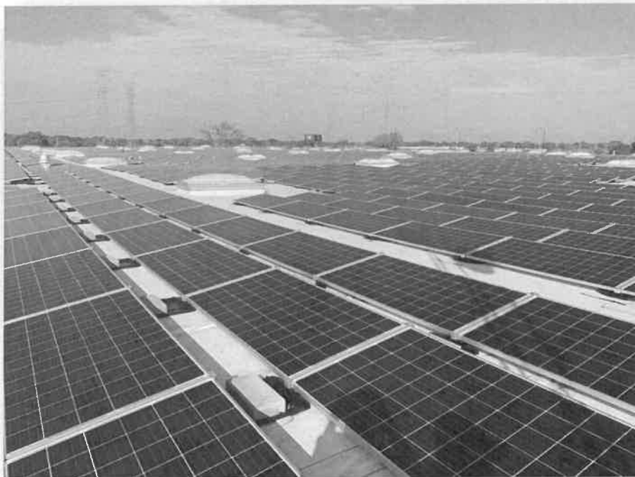
Roof Mounted in Illinois
