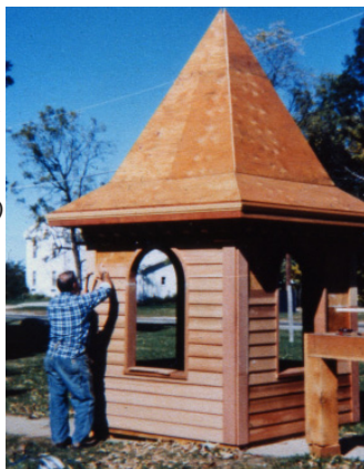
Stan Young works to finish the museum's new bell tower in the fall of 1980.
