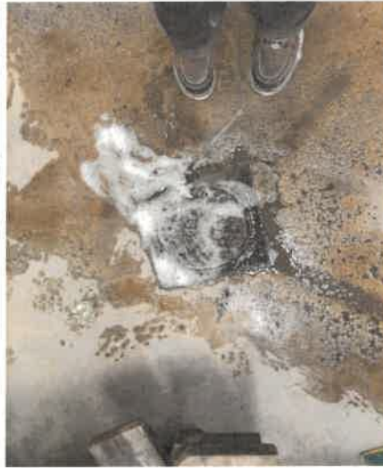
Floor drain to clean up any accidental spills.
