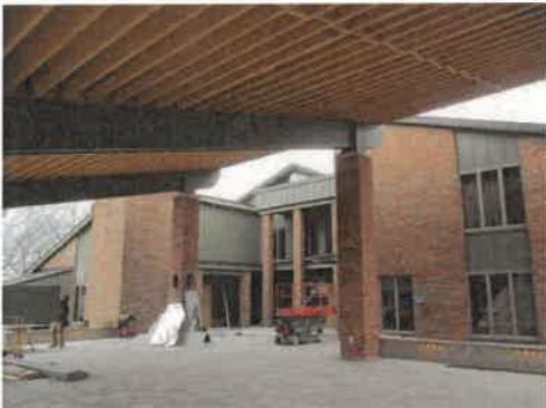
The roof of the pavilion at the Pickerill house will be fitted with solar panels to help power the all-electric building, seen here March 2, 2023. (Mark Foster)
