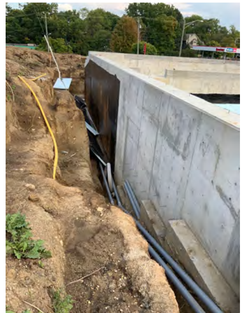
Conduit at North Wall.
