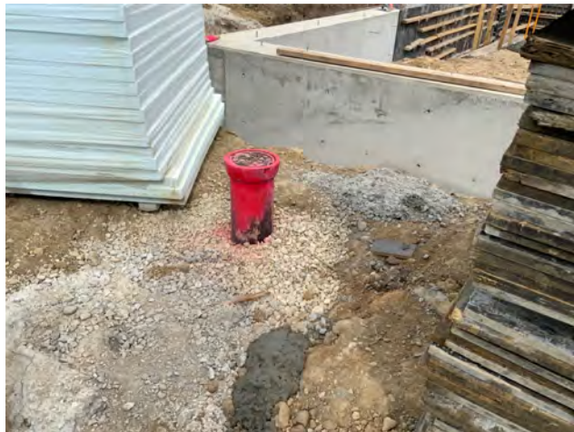
Underground Water Line
