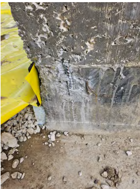
#3 - Exposed Rebar at 002B
