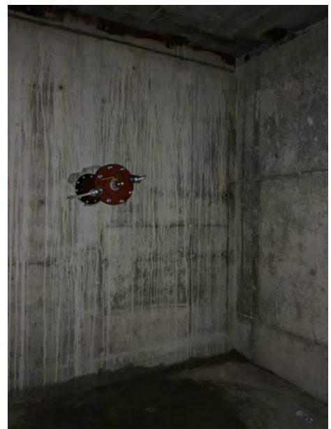
Incoming Water Line in Sprinkler
