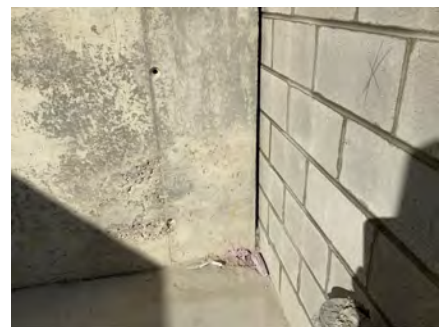
Gap between Conc. And CMU
