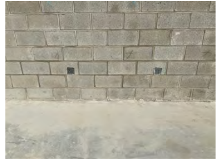
Recessed Electrical Outlets
