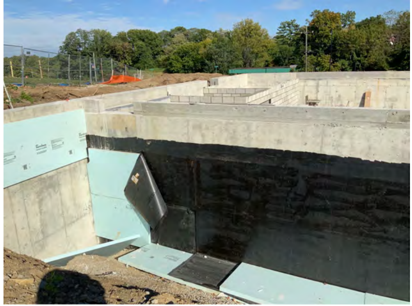
Opening for Door 106A Missing
