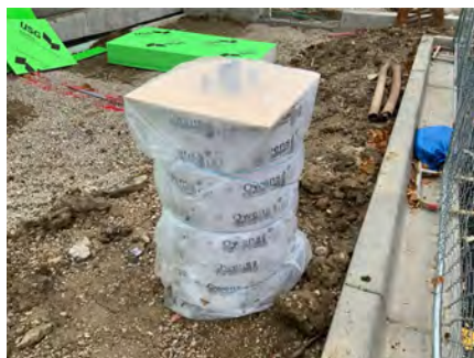
Light Pole Bases
