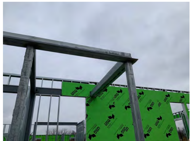
Bent Steel Angle at Entry
