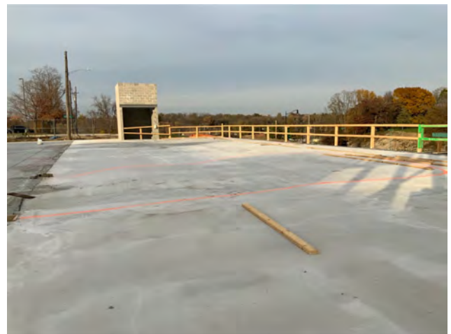
Self Leveling Damaged in Soft Area
