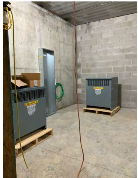
Electrical Equipment in Elec 003A
