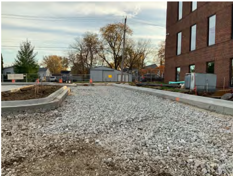
Curb and Gutter Shifted along West Side of Drive
