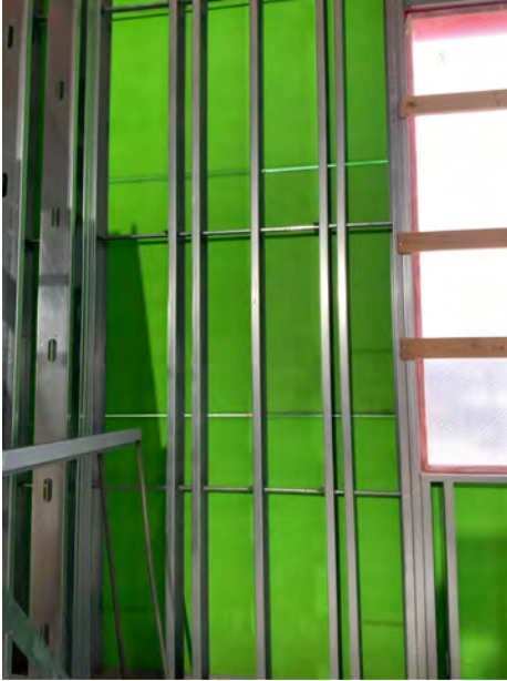
Gaps in Exterior Sheathing
