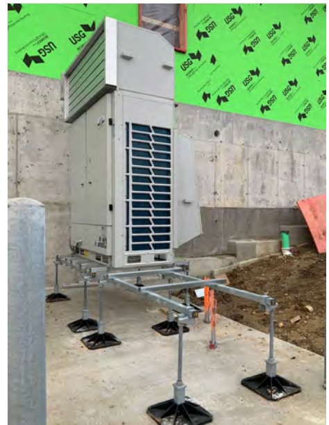
Mechanical Equipment on Rails
