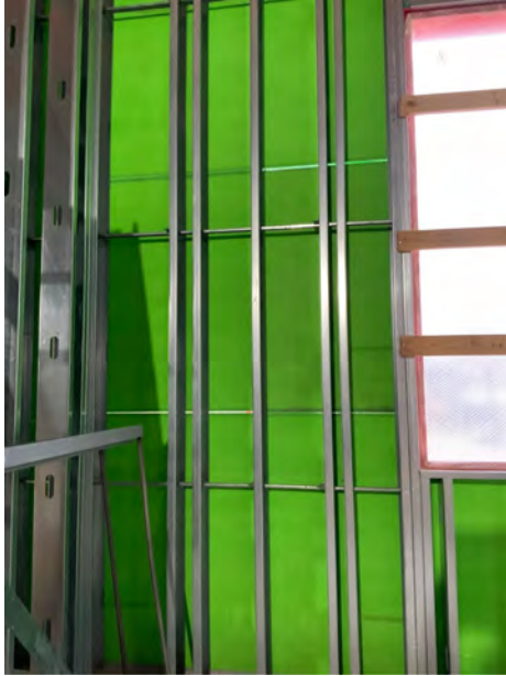
Gaps in Exterior Sheathing
