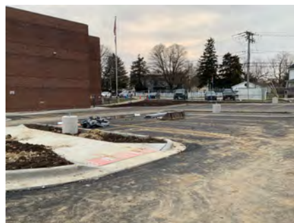
Site Lighting on West
