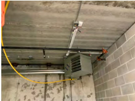
Unit Heater in Staging/Receiving
