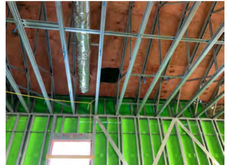
Ductwork to Exterior Louver
