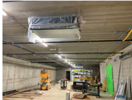
VRFs in Basement
