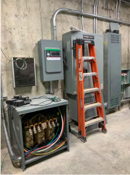
Electrical Equipment in Elec 003A
