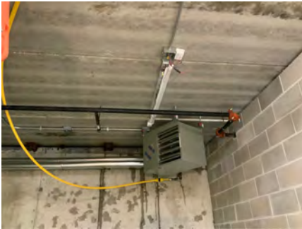
Unit Heater in Staging/Receiving
