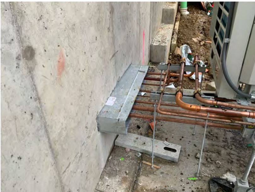
Pipe Penetrations for Outdoor Units
