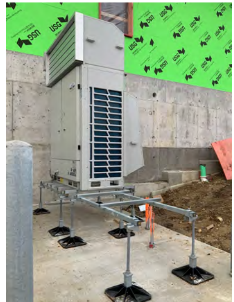
Mechanical Equipment on Rails
