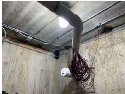
Sanitary Piping in Sprinkler Rm
