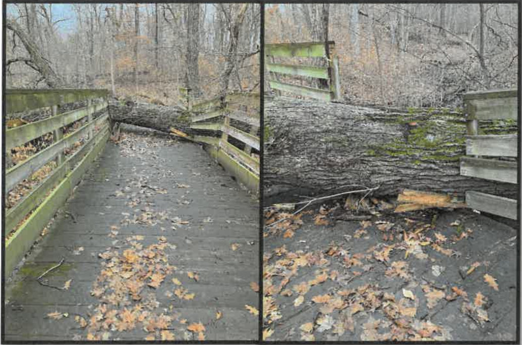
February tree fall event across a bridge at Harris Forest Preserve. Grounds crew removed tree and repaired damage to the bridge.
