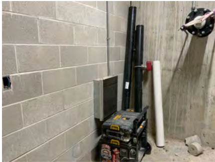
Wall Heater in Sprinkler
