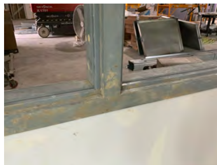
Dirt and Rust on HM Frame
