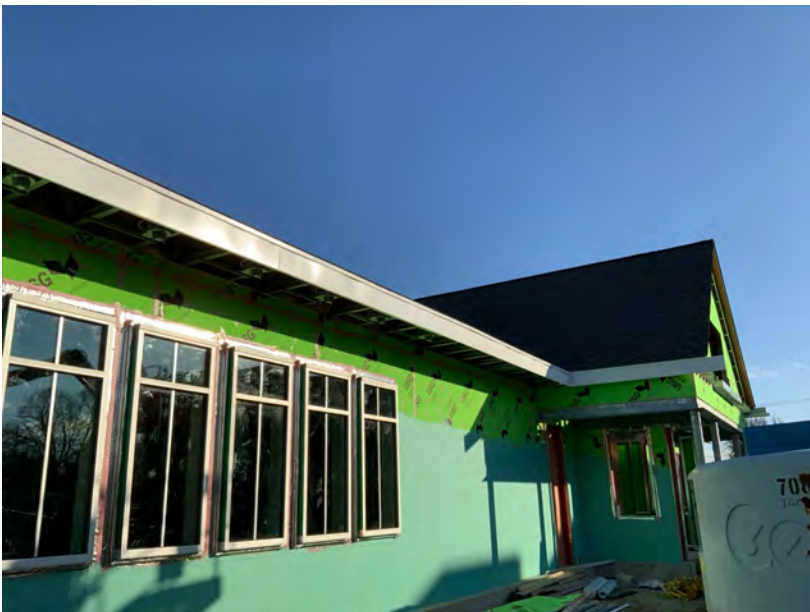
Aluminum Fascia showing Oil Canning
