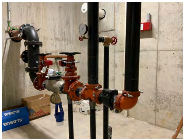
Water Riser in Sprinkler 005
