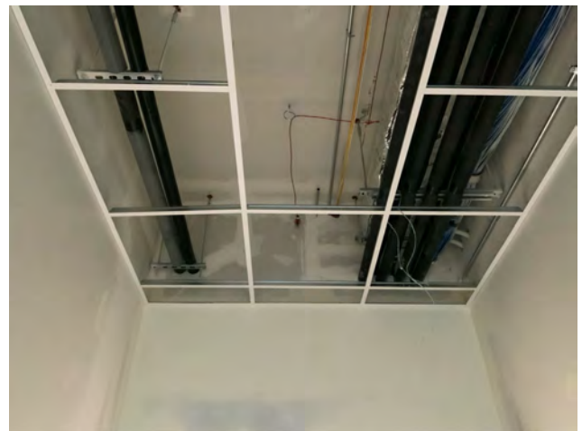
Thru Wall Penetrations Requiring Fire Caulking
