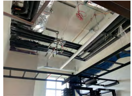
Ceiling Space in IT
