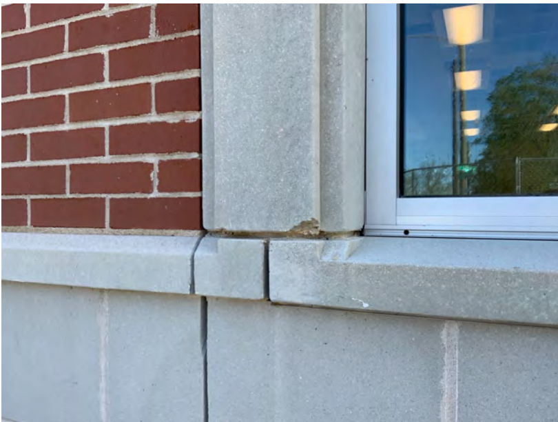
Cast Stone Jamb Damage on North
