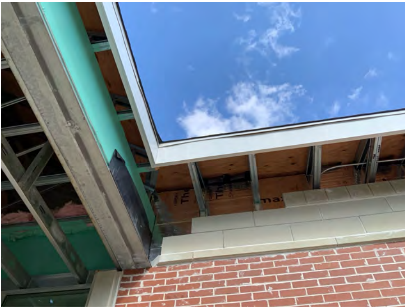
Bent Fascia Trim at Interior Corner of Entrance
