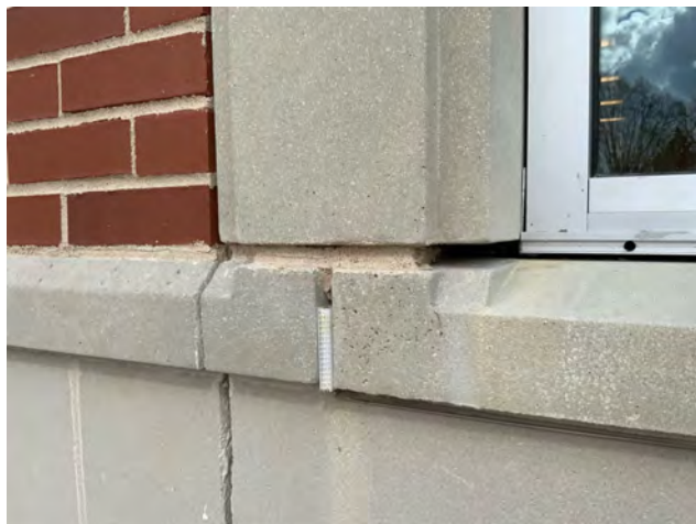
Mortar Missing at Cast Stone Jamb Base
