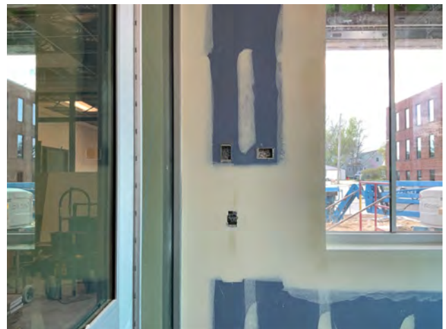
Electrical Power and Data for Monitor
