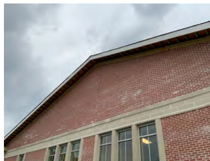
Weep Vents in Masonry
