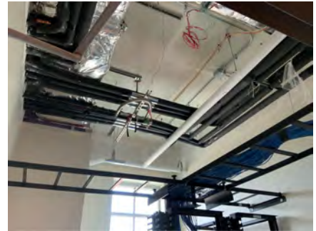
Ceiling Space in IT
