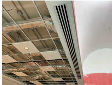
Mechanical Grille in Lobby
