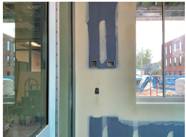
Electrical Power and Data for Monitor
