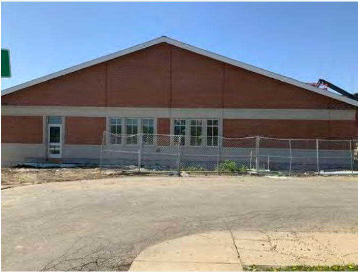
IMG_1742 Taken on Apr 22, 2024, 10:11 AM CDT Added on Apr 22, 2024, 3:10 PM CDT Added by Ken Gleason
