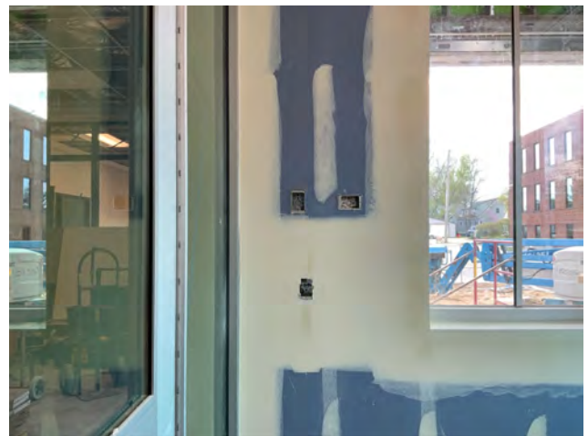
Electrical Power and Data for Monitor
