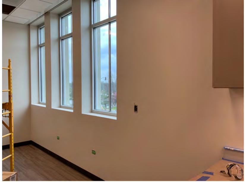
Window Shade Control in Break Room
