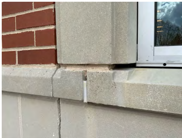
Mortar Missing at Cast Stone Jamb Base
