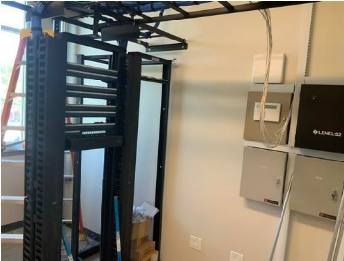
IT Room Taken on May 17, 2024, 3:57 PM CDT Added on May 17, 2024, 4:08 PM CDT Added by Ken Gleason
