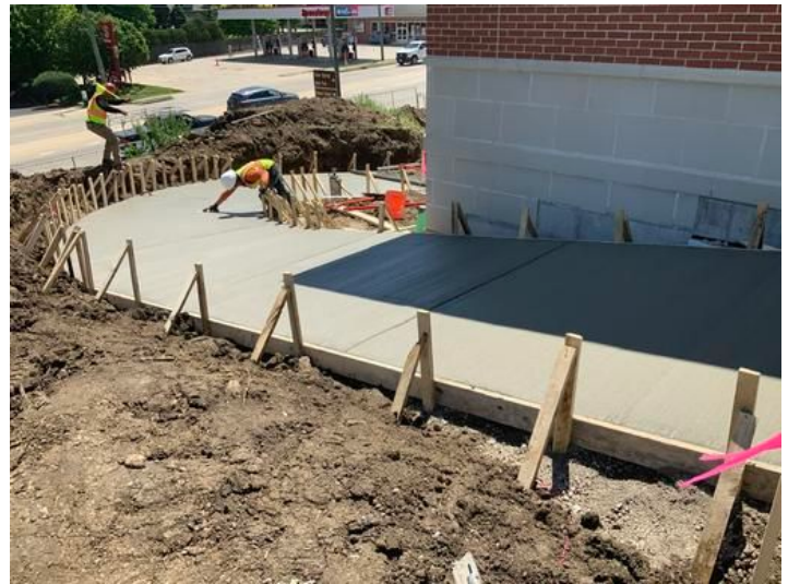
Drive Ramp NE Corner Taken on May 17, 2024, 12:13 PM CDT Added on May 17, 2024, 4:08 PM CDT Added by Ken Gleason
