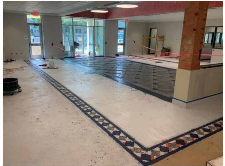
Lobby Terrazzo Flooring Taken on May 17, 2024, 3:56 PM CDT Added on May 17, 2024, 4:08 PM CDT Added by Ken Gleason
