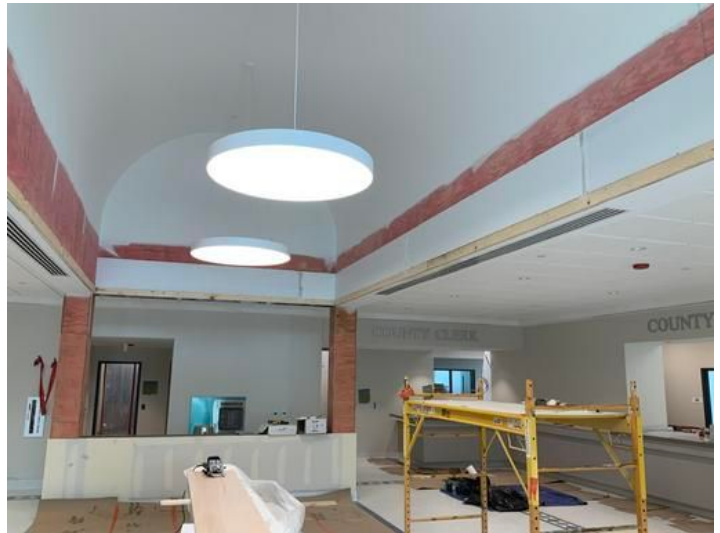
Flatstock trim being installed at lobby Taken on May 31, 2024, 3:16 PM CDT Added on May 31, 2024, 3:41 PM CDT Added by Ken Gleason
