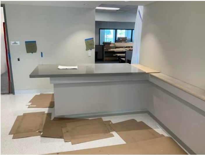
Countertop install at lobby Taken on May 31, 2024, 3:17 PM CDT Added on May 31, 2024, 3:41 PM CDT Added by Ken Gleason
