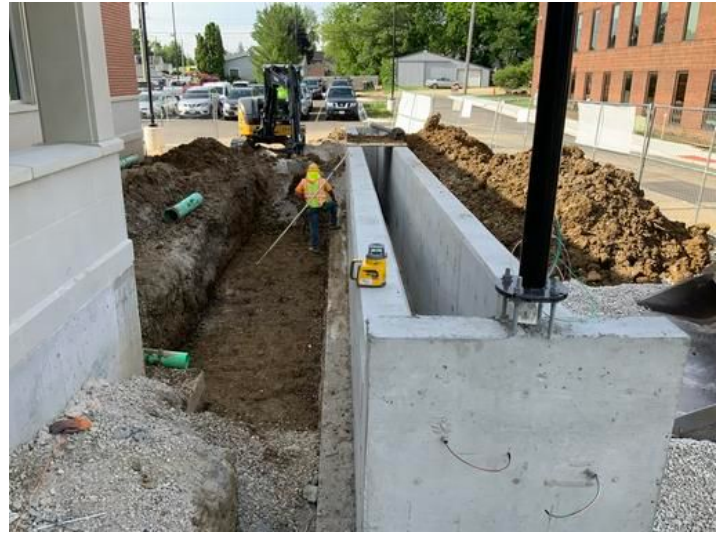
Planter box & excavation Taken on May 31, 2024, 8:25 AM CDT Added on May 31, 2024, 3:41 PM CDT Added by Ken Gleason
