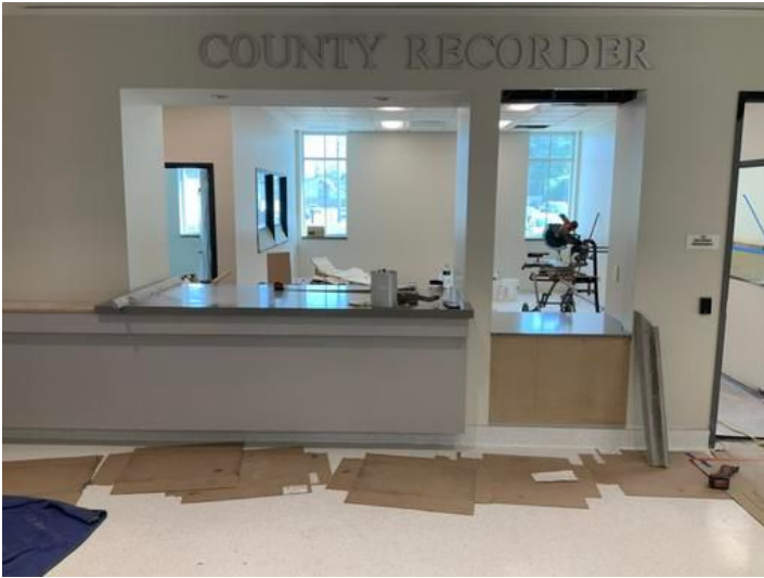
Countertop install in lobby Taken on May 31, 2024, 3:17 PM CDT Added on May 31, 2024, 3:41 PM CDT Added by Ken Gleason
