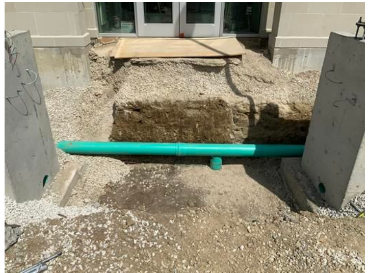
Roof drain tile being installed Taken on May 31, 2024, 3:13 PM CDT Added on May 31, 2024, 3:41 PM CDT Added by Ken Gleason
