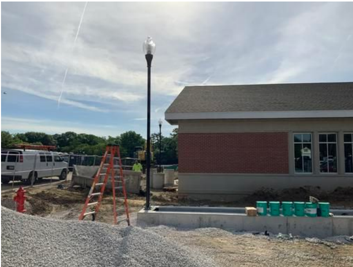
Exterior site lighting Taken on May 31, 2024, 8:42 AM CDT Added on May 31, 2024, 3:41 PM CDT Added by Ken Gleason
