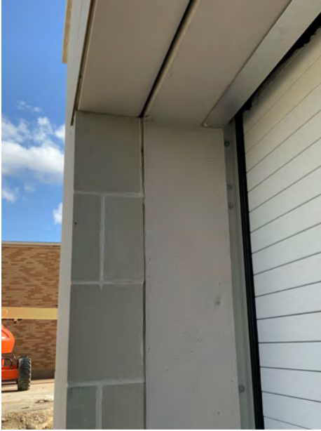
Paint Color at Concrete Jamb
