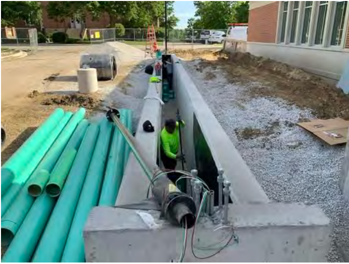
Planter box with waterproofing work Taken on May 31, 2024, 8:25 AM CDT Added on May 31, 2024, 3:41 PM CDT Added by Ken Gleason
