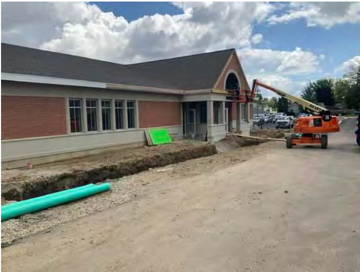
Front Entry Flat Roof Taken on May 10, 2024, 12:58 PM CDT Added on May 10, 2024, 1:17 PM CDT Added by Ken Gleason
