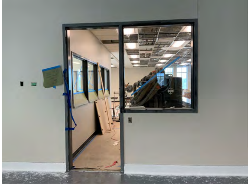
Electrical Box at Door Frame 104A
