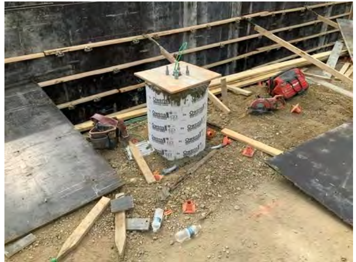
Exterior Lighting Base
