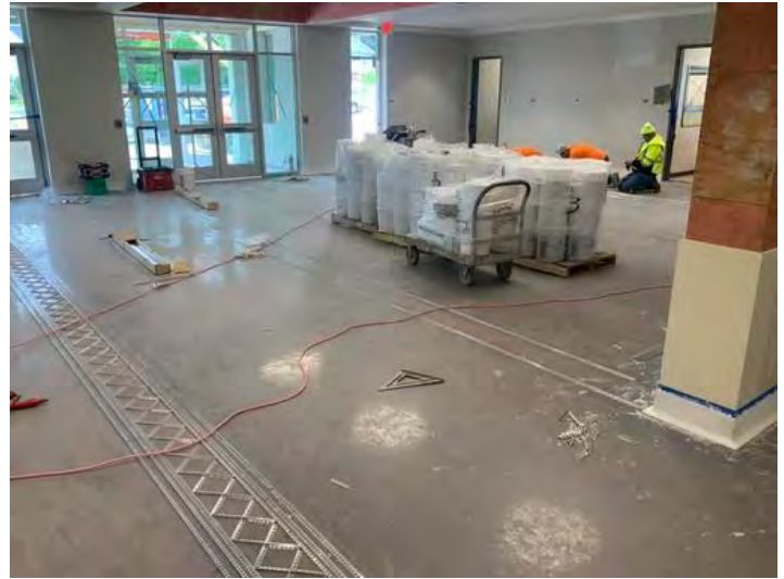
Lobby Terrazzo Tracks Taken on May 10, 2024, 1:03 PM CDT Added on May 10, 2024, 1:17 PM CDT Added by Ken Gleason
