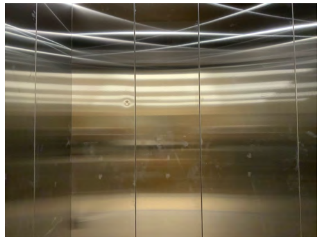
Dented Panel in Elevator
