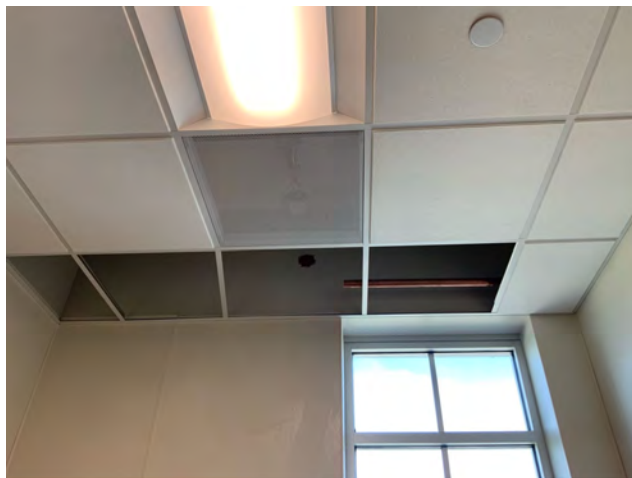
Condensate Pipe in JC
