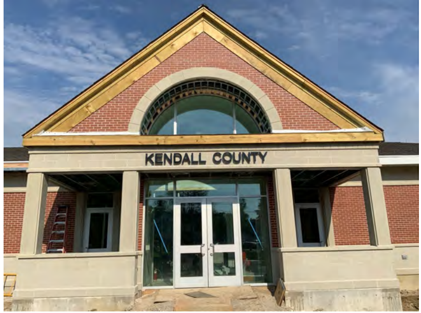
Kendall County Halo Lit Sign and Trim Boards
