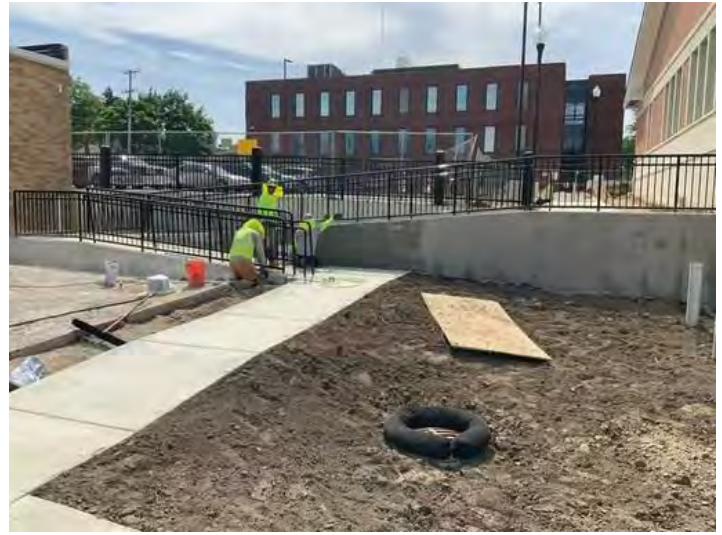
Rubbed finish install at ADA ramp Taken on May 31, 2024, 3:26 PM CDT Added on May 31, 2024, 3:41 PM CDT Added by Ken Gleason
