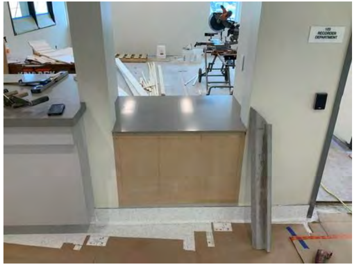
Counter top install at lobby Taken on May 31, 2024, 3:17 PM CDT Added on May 31, 2024, 3:41 PM CDT Added by Ken Gleason
