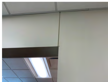
Control Joint in Break Room
