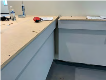
Interior Corner Gap at Reception
