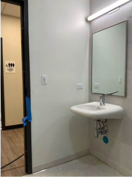
Wall in Toilet Room
