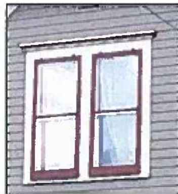
Wood storm windows are not only attractive but they increase energy efficiency as well.
