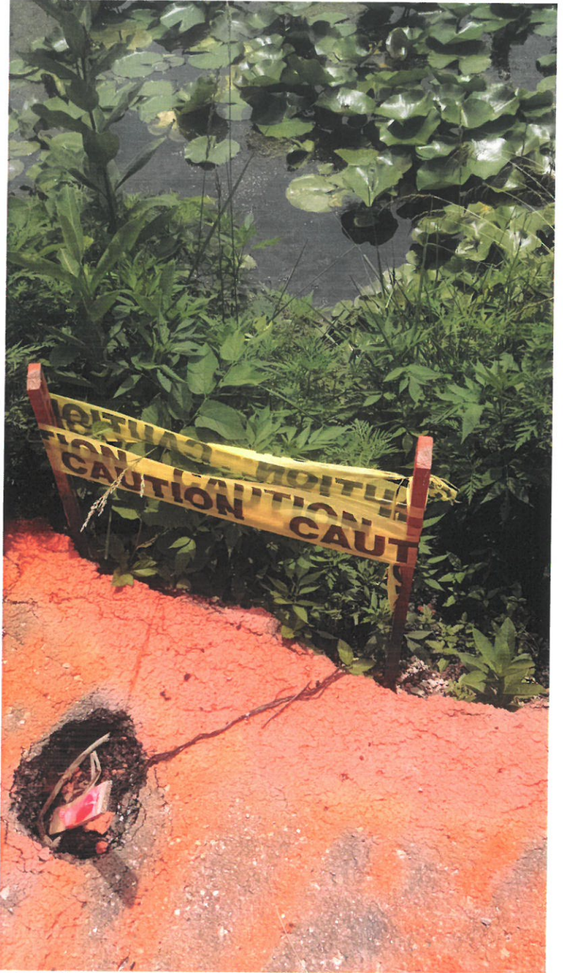
Pond shoreline erosion road undercut
