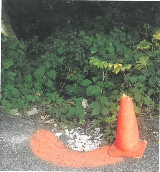
Drainage outlet erosion road undercut
