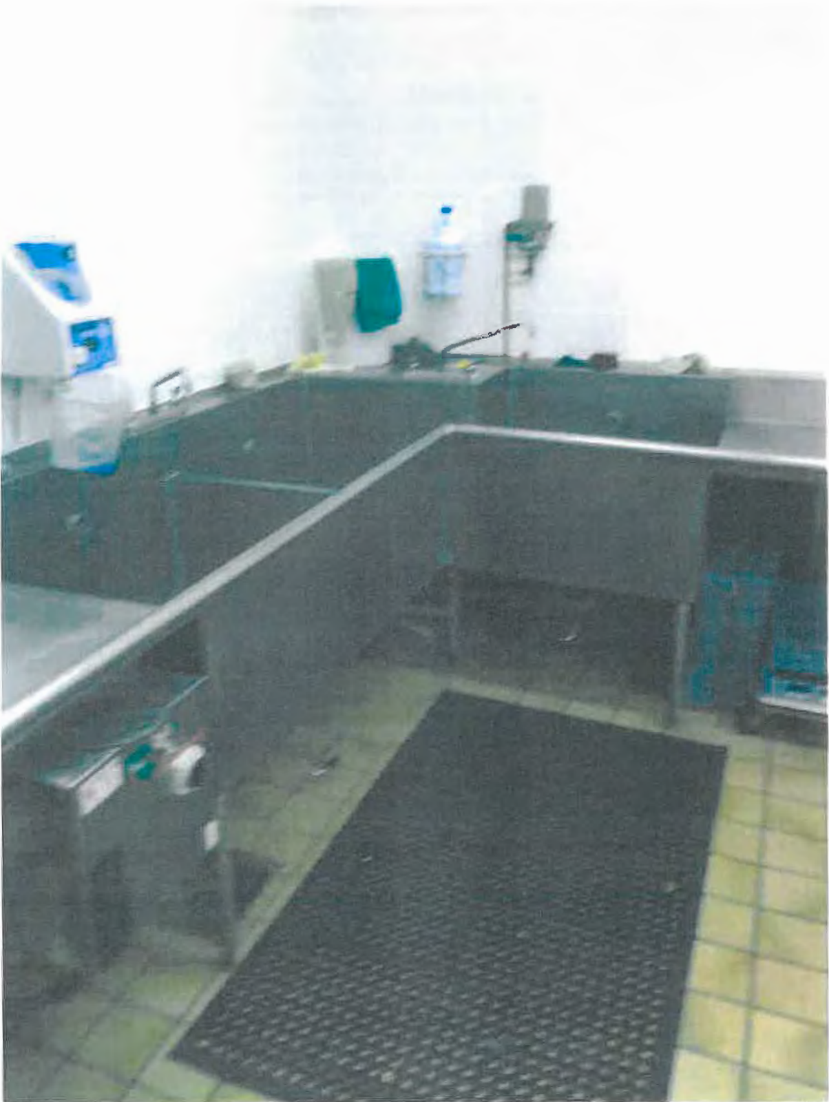
3 station wash sinks
